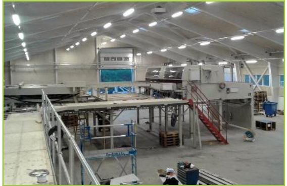
Installation of the layer crosscut & stacking line No. 1 at DTE A/S
